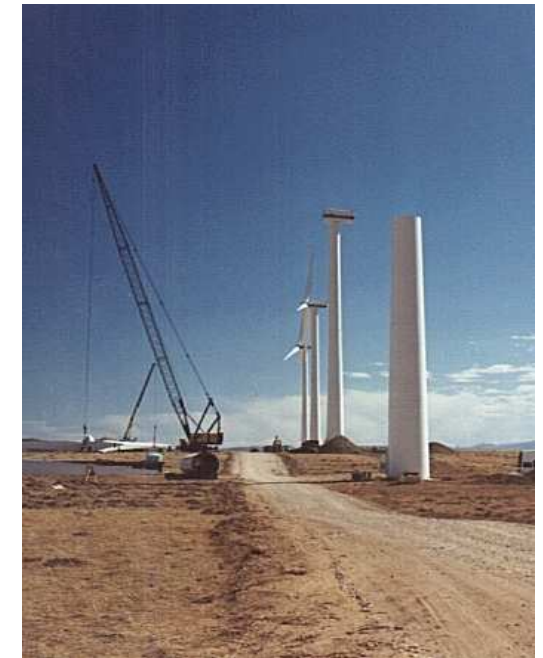
Vestas turbines under construction at the Medicine Bow site. The turbines are now operational.
