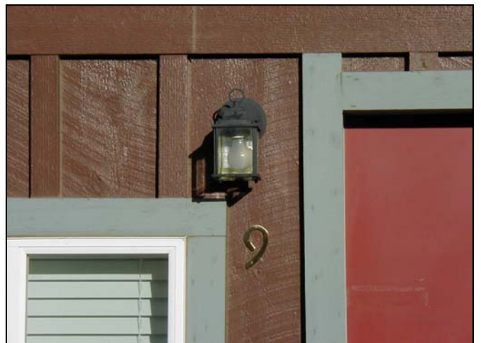
Not code compliant—bulb is visible
