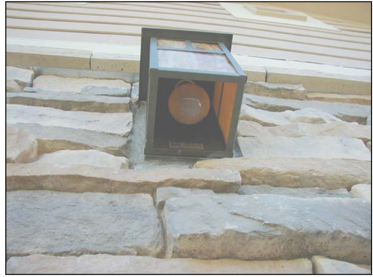
Code compliant—bulb is shielded and downcast
