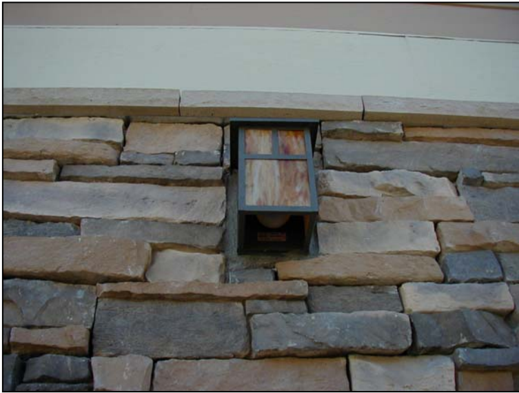
Code compliant—bulb is shielded and downcast
