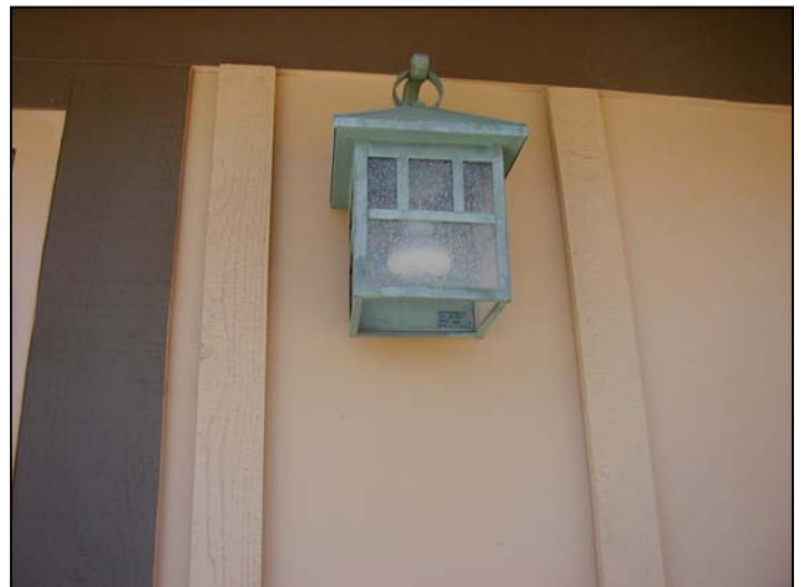
Not code compliant—bulb is visible
