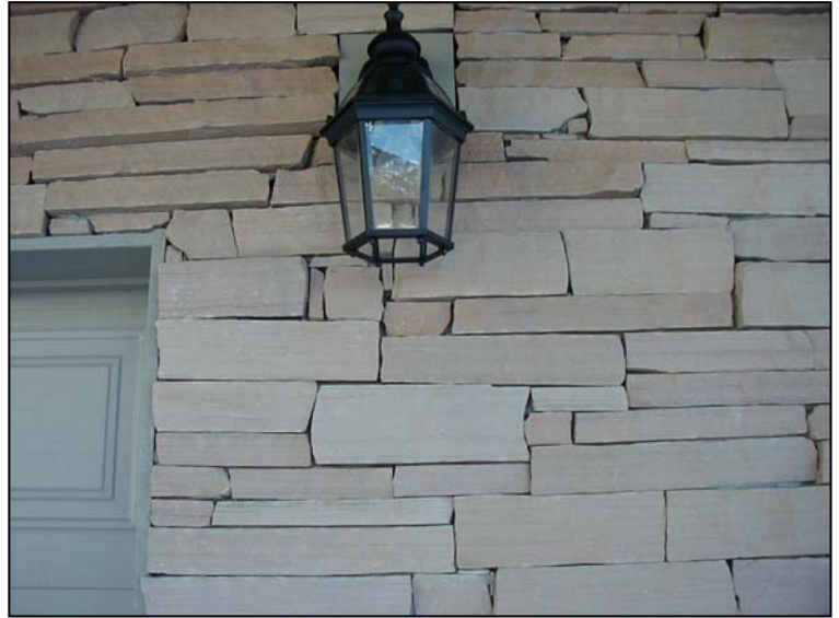
Not code compliant—bulb is visible
